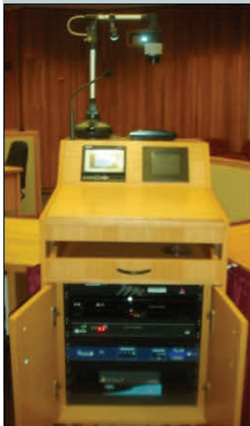
Podium/Lectern with document camera, DVD Combo Unit and inputs for laptops utilized by attorneys.
